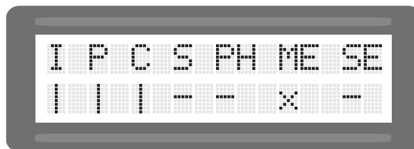
Impulse-, pedestrian - and close button not triggered. STOP-button and photocell are triggered. Contact strip (main closing edge) not connected or defect. contact strip (side closing edge) triggered.
